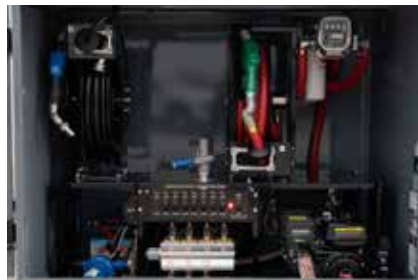
Utility Box Shown with Diesel & DEF
